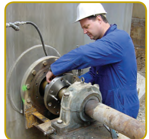
INSTALLING THE 4.5 IN. FULLY SPLIT EA TYPE-1 SEAL ON BLACK LIQUOR AGITATOR.
