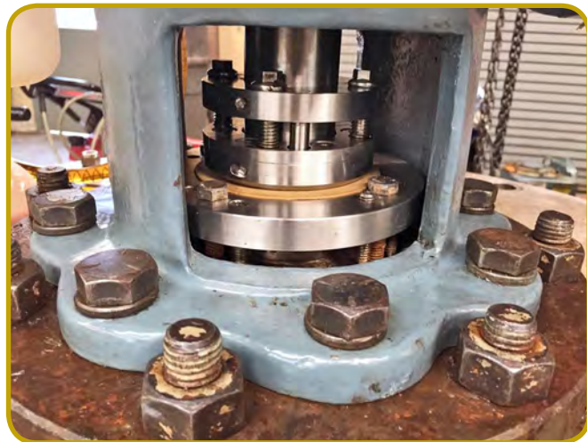
2" OFS TYPE-1 SEAL INSTALLED ON A TOP-ENTRY AGITATOR CONTAINING VOCs AND MOLTEN PLASTIC RESIN
